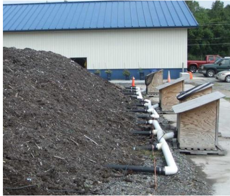
Amboy Compost Site Aerated Static Pile System
