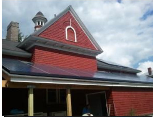
Preble Town Hall with 9 kW solar PV panels installed on roof
